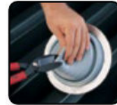
1. Choose pipe opening and trim
